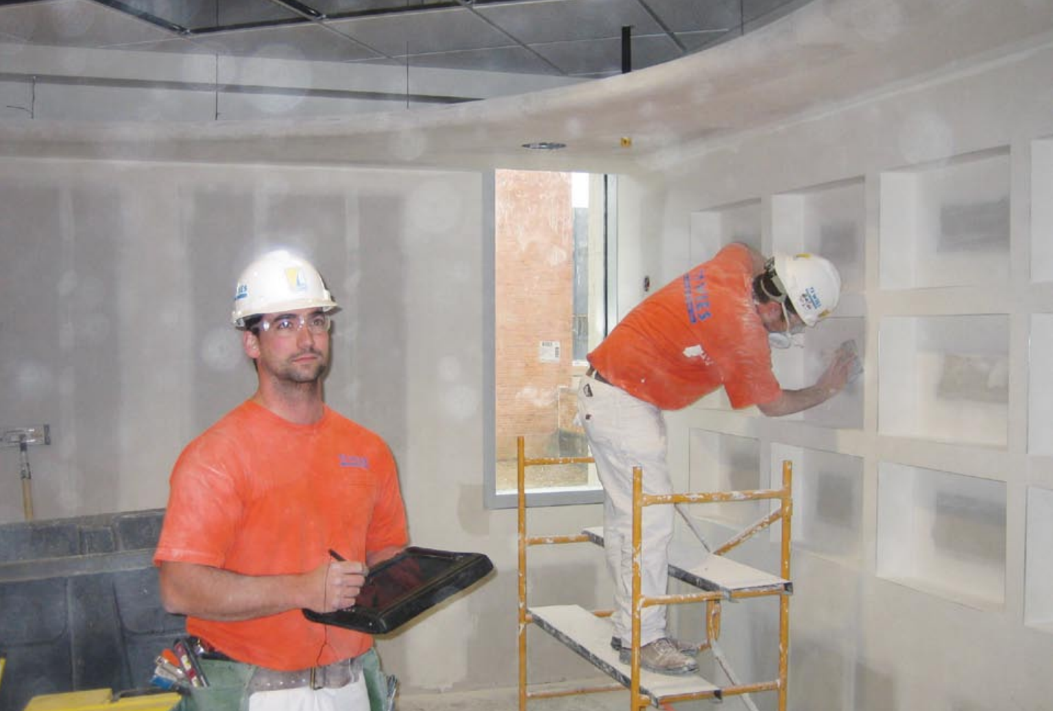
Jason Fields, Carpenter and General Foreman, T.J. Wies Contracting, uses the DPC tablet to track jobs electronically. In one instance, the company recouped $199,000 in potential cost overruns.
